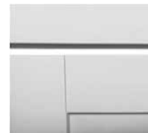
Representative of acceptable joint fracture
